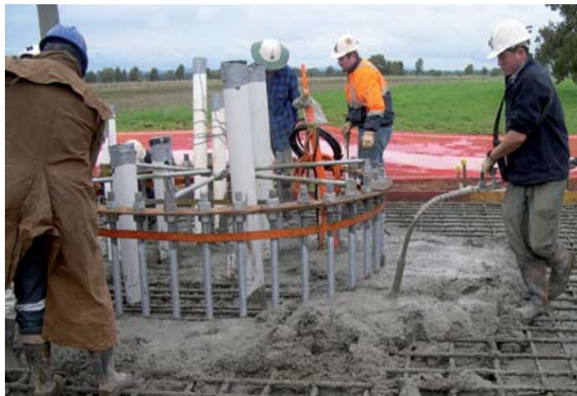
Pouring concrete for the foundation of the 12m ASKAP test antenna at the Parkes Observatory. Photo Barry Turner
